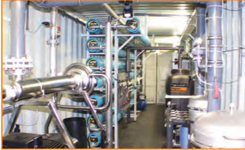
Sea water desalination 500 m 3 /day
