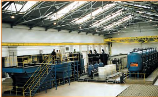
Water works 5.000 m 3 /day
