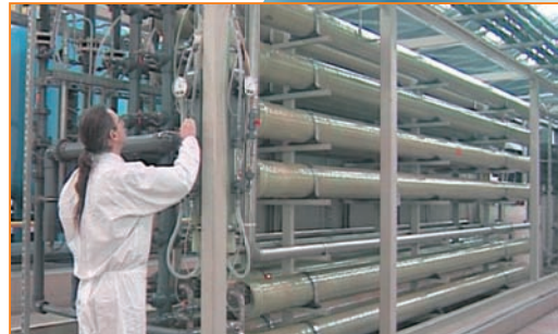
Reverse-osmosis 3.000 m 3 /day
