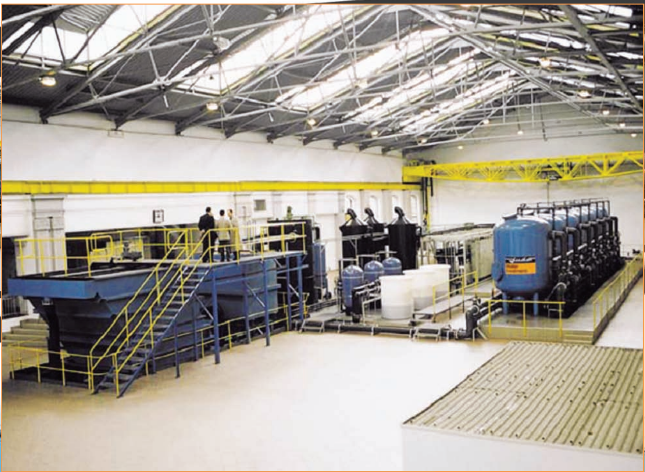
Customized plant in overview
