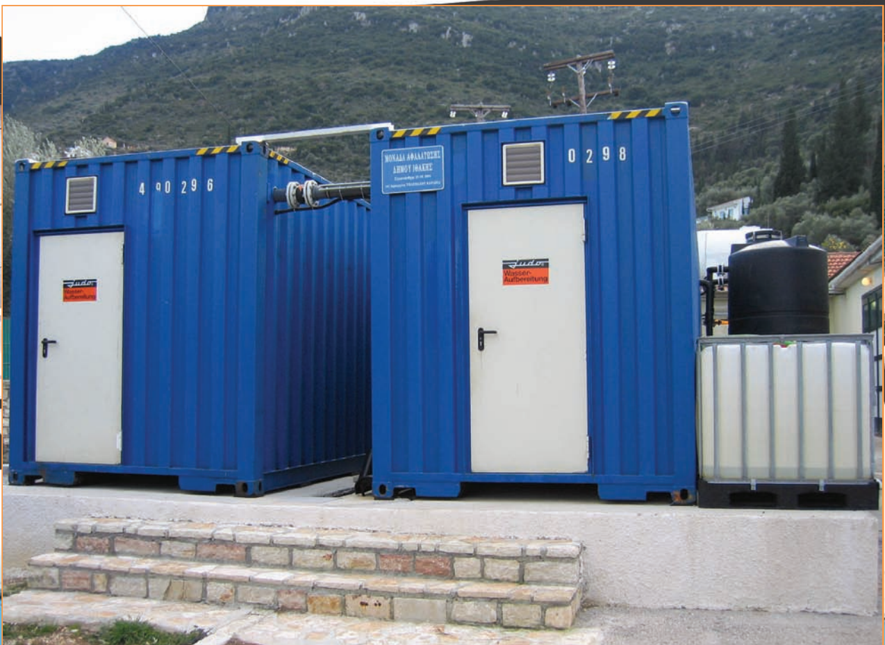
Seawater desalination in Vathi
