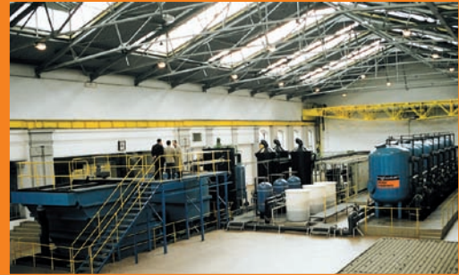
Water works 5.000 m 3 /day
