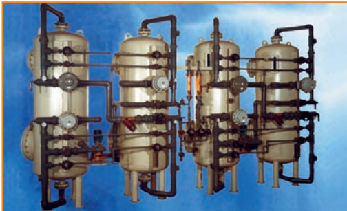
Decarbonization and softening by ion-exchange
