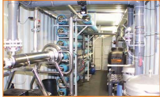
Seawater desalination 500 m 3 /day
